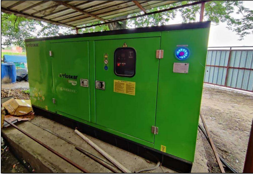
Annexure 7: Photograph showing DG set
